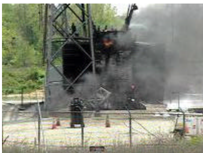
Hours after the fire, the substation continued to smolder
