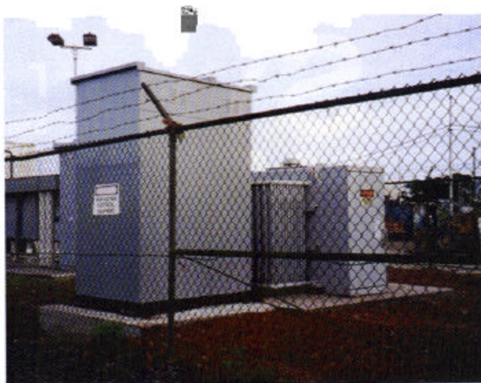
Partial discharge testing not only helps head off costly transformer catastrophes, it's an important complement to preventive maintenance.
